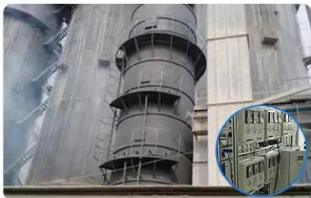
— Acid alkali waste tower —
